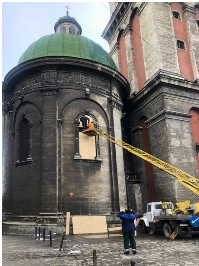
Workers on a crane securing a stained-glass window in the apse of the Dormition Church (1591–1629) in Lviv on February 28, 2022. Photograph by Iryna Horban.
